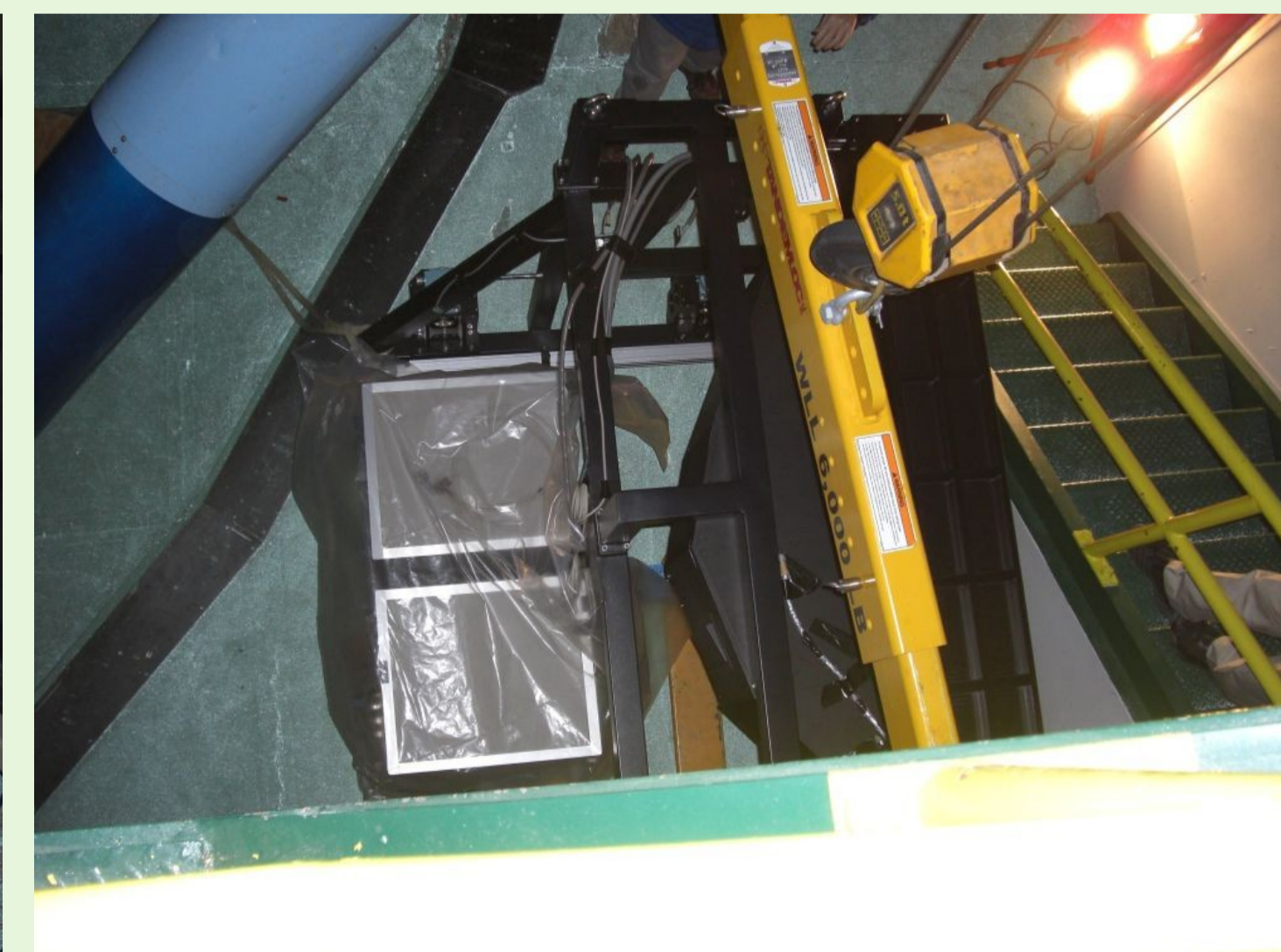
Test to move the mount with a crane between the Cassegrain floor (standby) and the Nasmyth floor.
